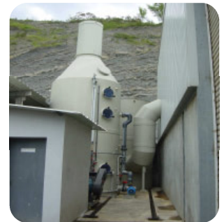
Exit of the deodorization facility
